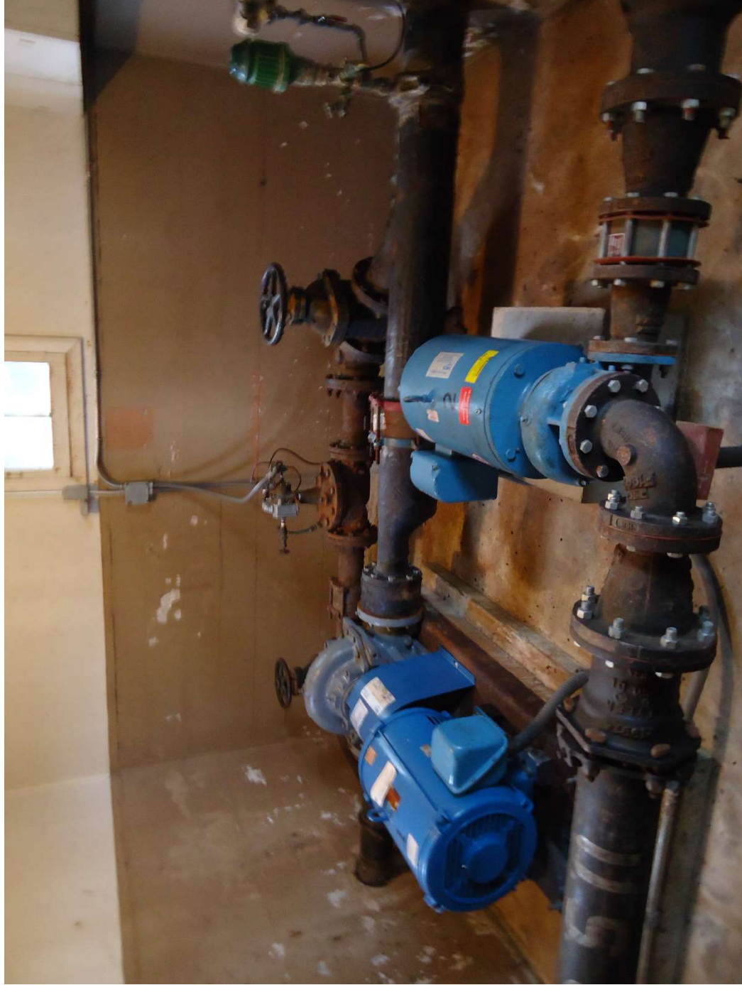
BUTLER BOOSTER PUMP STATION
