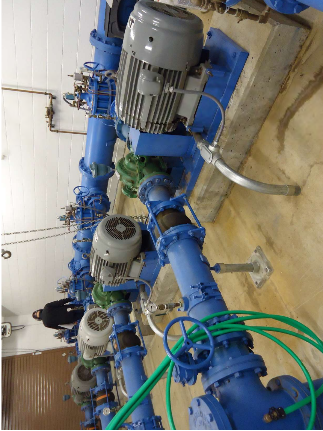
ANGELO BOOSTER PUMP STATION
