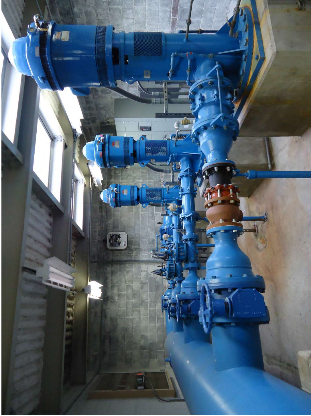
LACAMAS BOOSTER PUMP STATION
