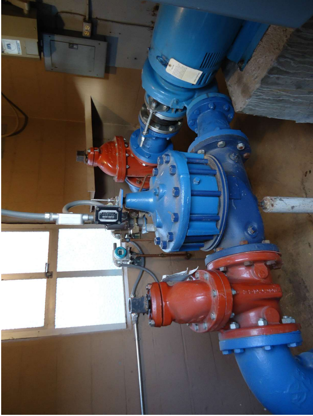
FOREST HOME BOOSTER PUMP STATION
