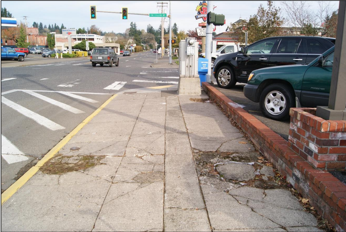
Figure 2: Example of damaged sidewalk that is a barrier to the disabled
