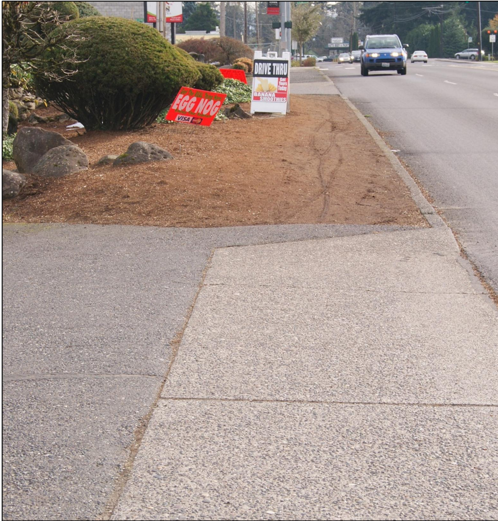
Figure 6: Examples of existing missing sidewalk section
