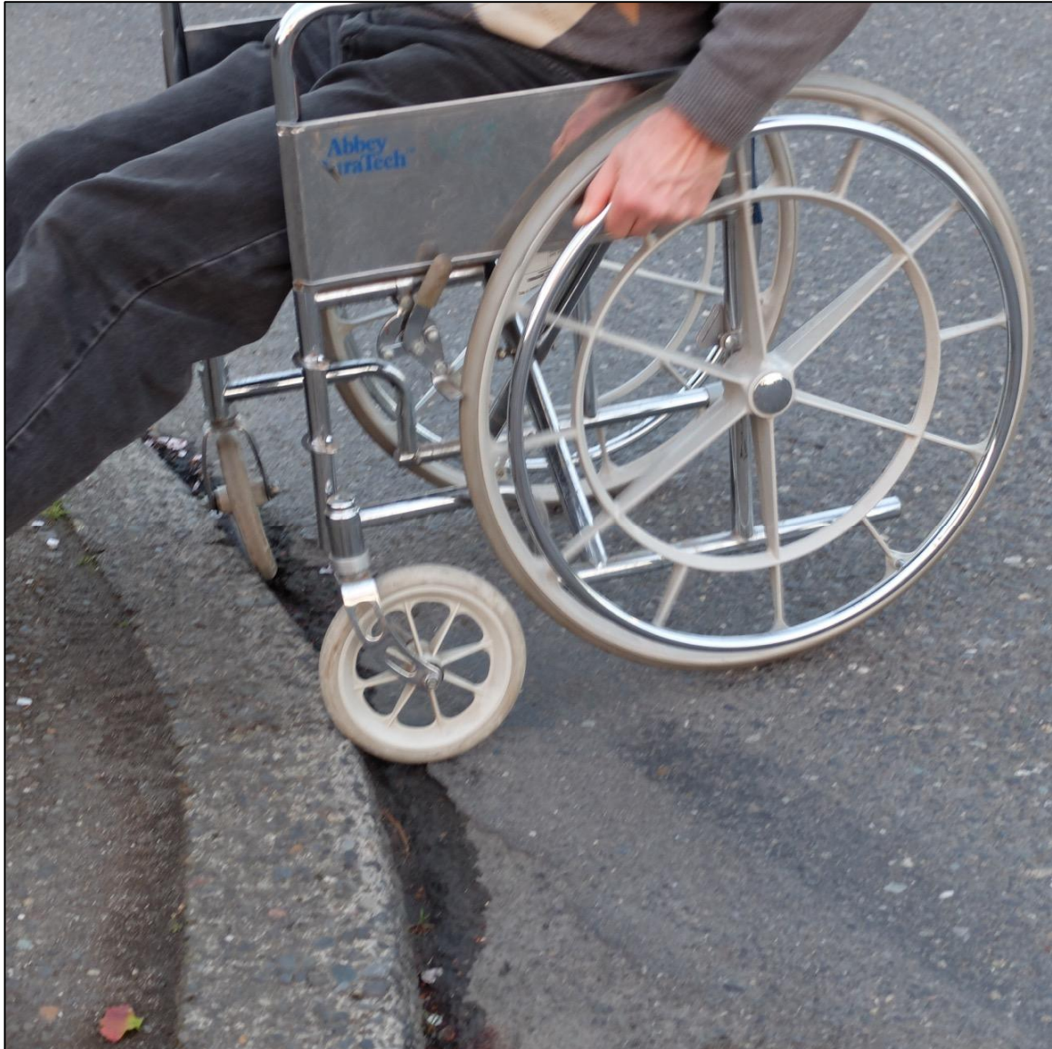
Figure 1: Example of ramp lip of gutter that is a barrier to the disabled
