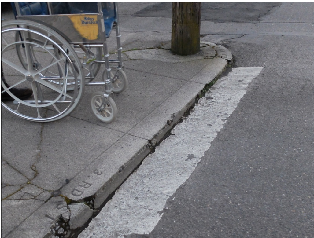
Figure 3: Example of full height curb that is a barrier to the disabled
