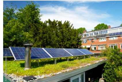
Solar panels on a green roof (Source: © René Notenbomer/ Adobe Stock)
